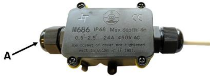
Figure 3 – Junction box A – Cable connection point
